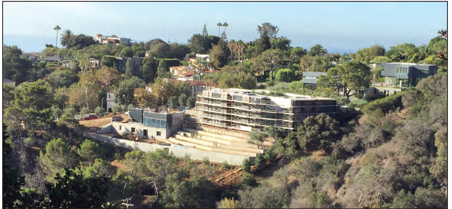
This single-family residence, under construction, is off Los Liones Drive in Pacific Palisades.
